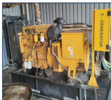
Backup power for safety-critical systems
