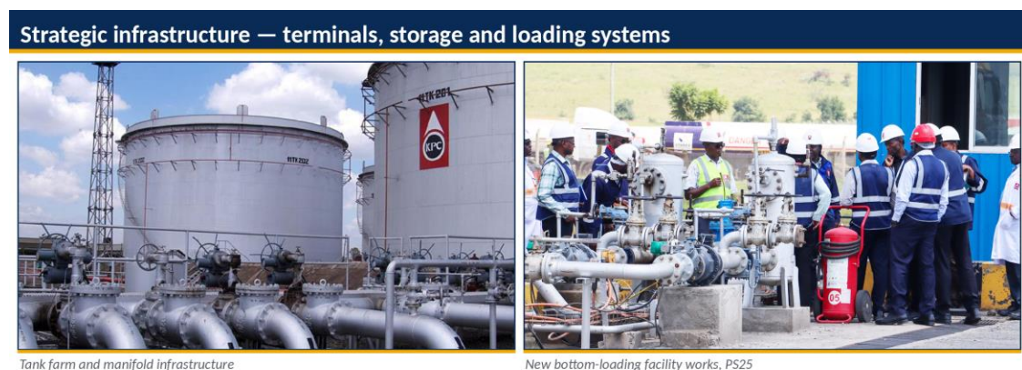
Figure 4: Strategic storage and loading infrastructure
