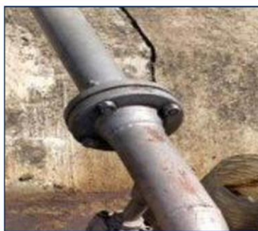
Spill-control bunding, PS14
