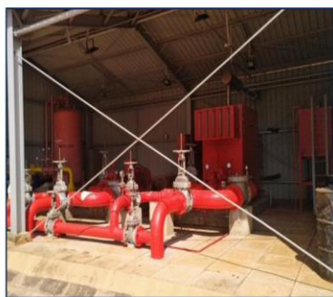
Fire suppression distribution, PS3
